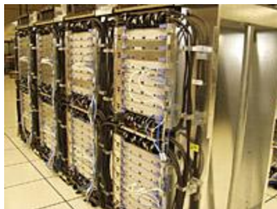
The world's most powerful supercomputer, BlueGene/L, is installed at Lawrence Livermore National Laboratory.
